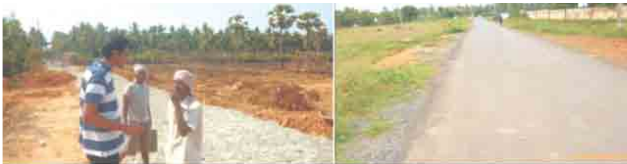
Efforts of Team NIFTEM under VAP leading to construction of Pukka Road in village Kalavacharla, Rajahmundry/East Godavari, Andhra Pradesh
